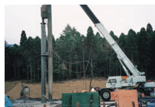
Geothermal, Oil Well Surface drilling down to 50m in depth for geothermal and oil well.
